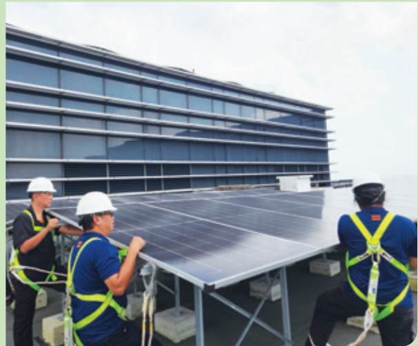
Solar panels installed at MBC.
