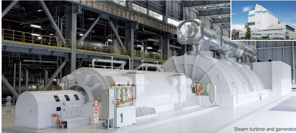
Steam turbine and generator
