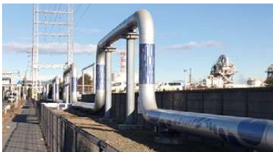
Steam supply pipe
