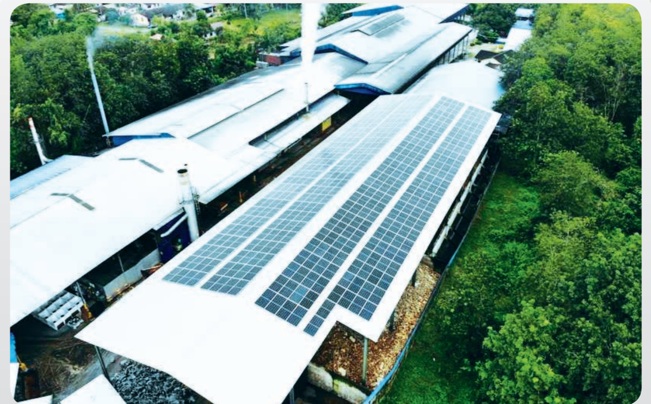
Aerial view of solar panels installed in Euroma factory in Kedah, Malaysia.
