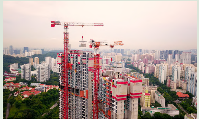
Prefabricated concrete modules were prefinished with tiles, cabinetry and more, before they were transported to the site of Avenue South Residence to be hoisted and stacked on top of one another. Photo: United Tec Construction
