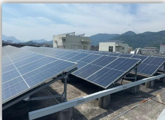
Yamada's Photovoltaic System
