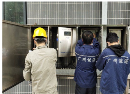
>>> Completion of the annual third-party inspection of totalizer and pressure transmitter among other measuring instruments
