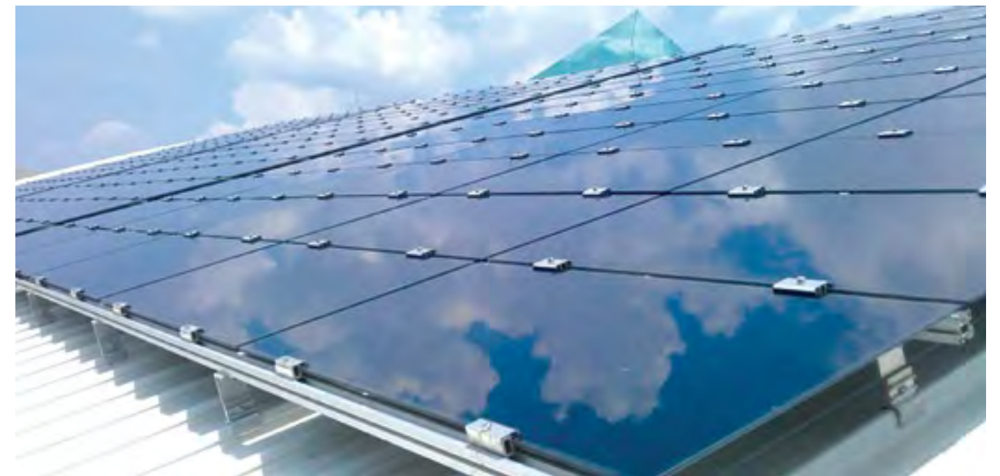
Solar System Project in hospitals across Malaysia.
