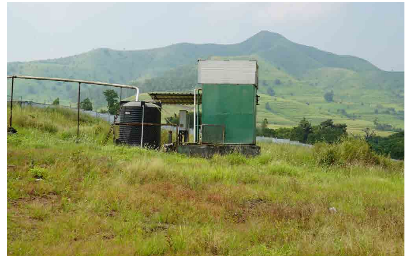
Waste Incinerator, Japfa India
