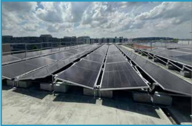
Installed Solar Panels
