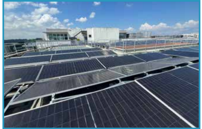
Installed Solar Panels
