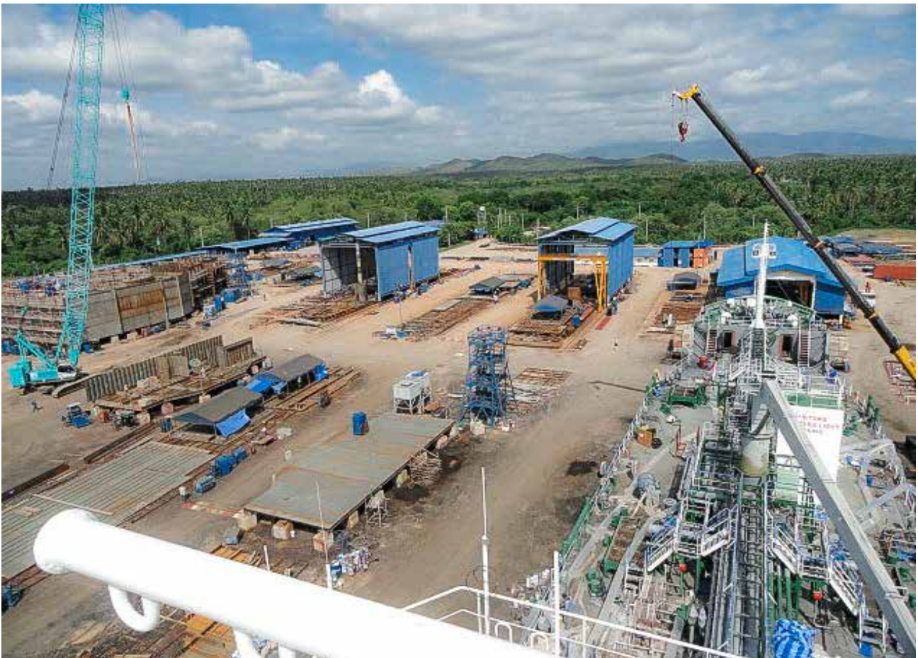
Above: Our shipyard in Thapsakae, Thailand, with 70,000 sqm of land space to undertake EPC projects and provide new building services such as offshore modules and oil rigs structures. We have successfully completed two EPC projects in this shipyard, and have successfully launched and delivered them to our customers.
