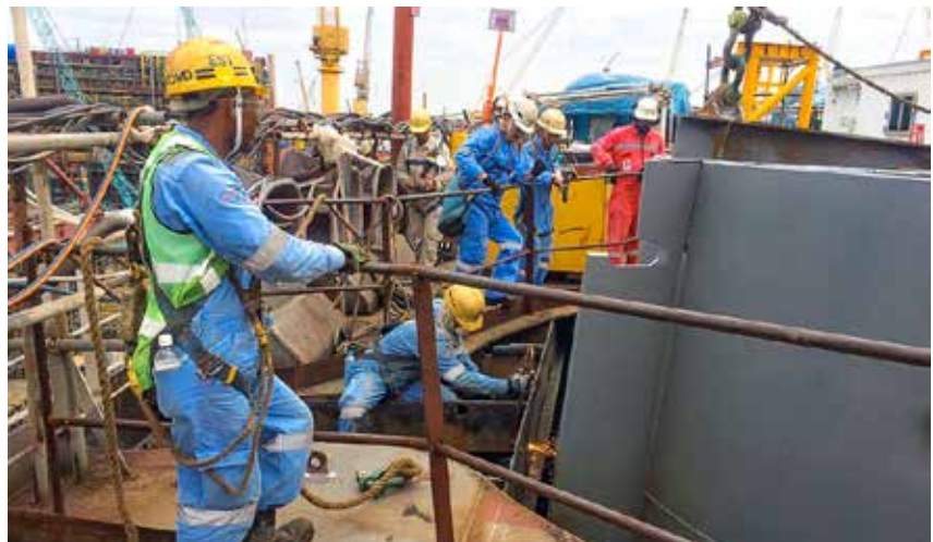
Above: A worker welding, with a team of supervisor and safety officers doing their safety inspection rounds. All of them had donned their safety equipment.
