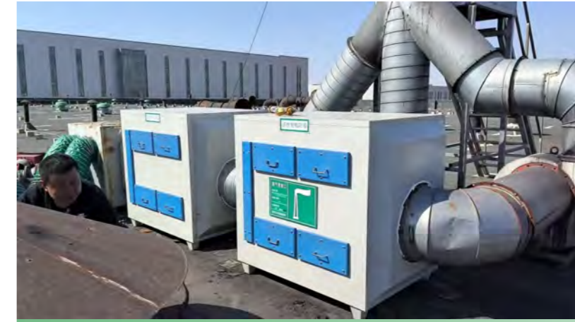
VOC Environmental Equipment Upgrade
