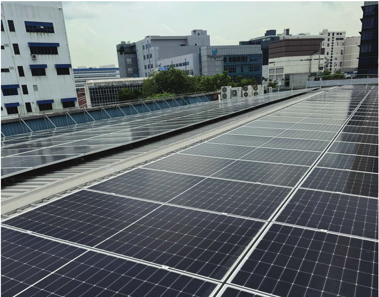
New solar panels installed at QAF Fruits which became operational in FY2024.
