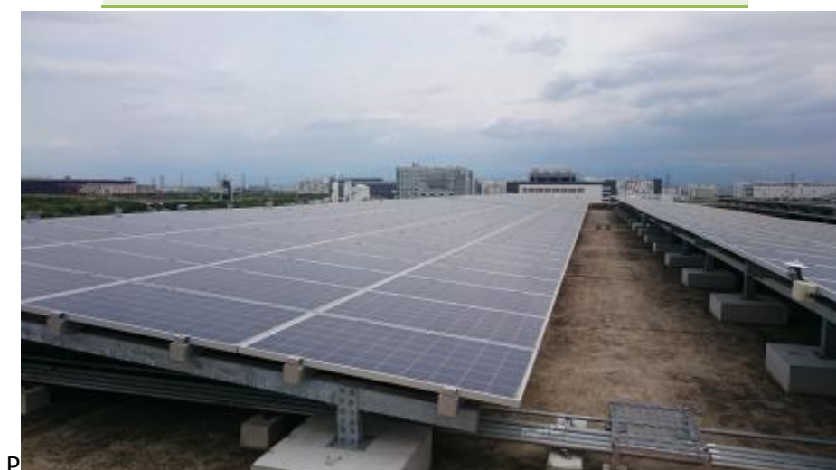
CMMT Solar Panel modules at Roof
