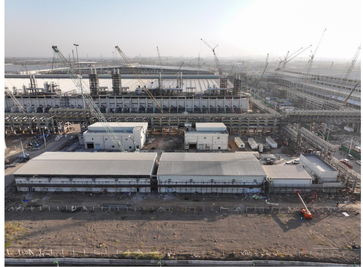
Chemical Storage Area
