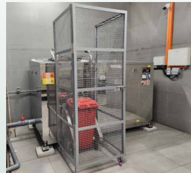
"Food waste biodigester" installed at Funan commenced its pilot in late 2022
