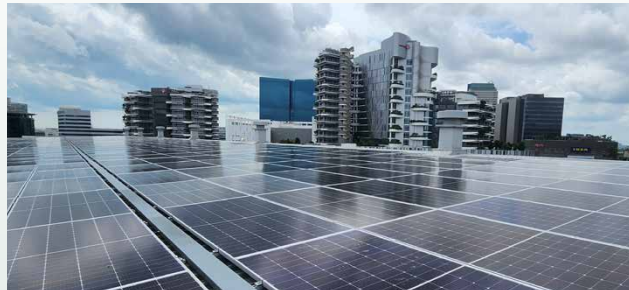
Tapping on renewable energy with solar panels installed on the rooftop of IMM Building
