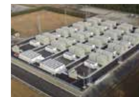
Buzen Battery Storage and Transformer Station
