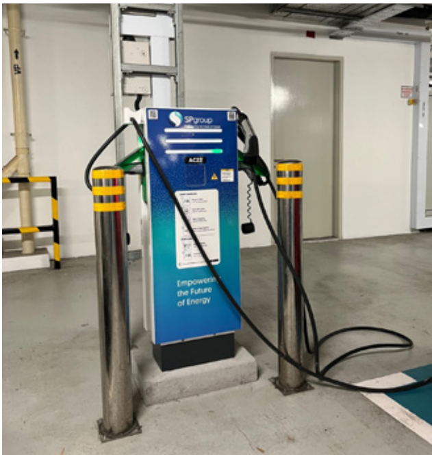
Electric vehicle charging station at Paya Lebar Square
