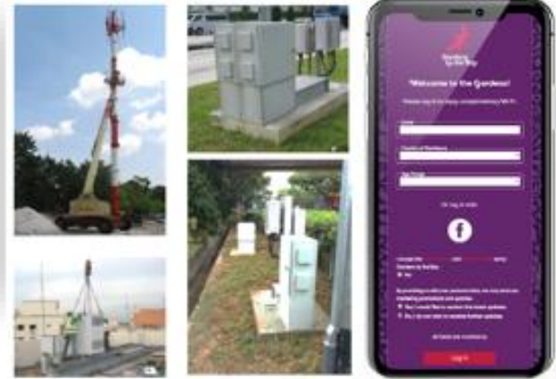
5G and WiFi Infrastructure
