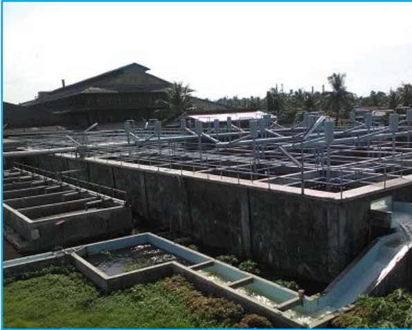
Waste water treatment plant
