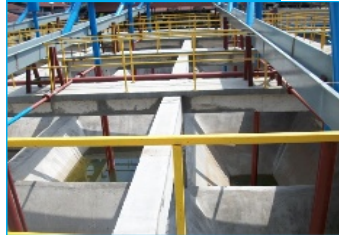
Waste water treatment plant
