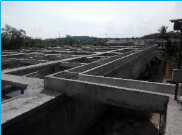
Waste water treatment plant
