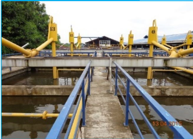
Waste water treatment plant
