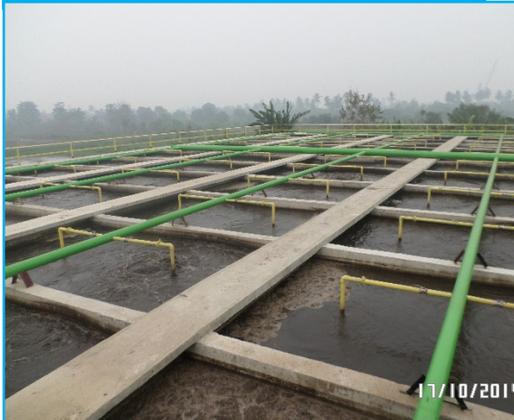
Waste water treatment plant
