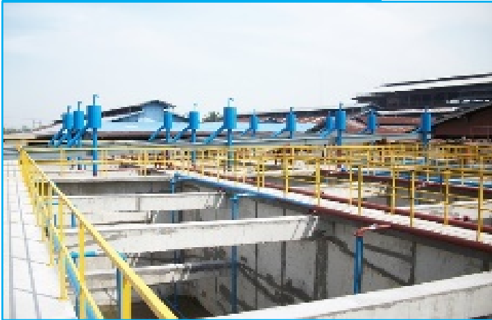
Waste water treatment plant
