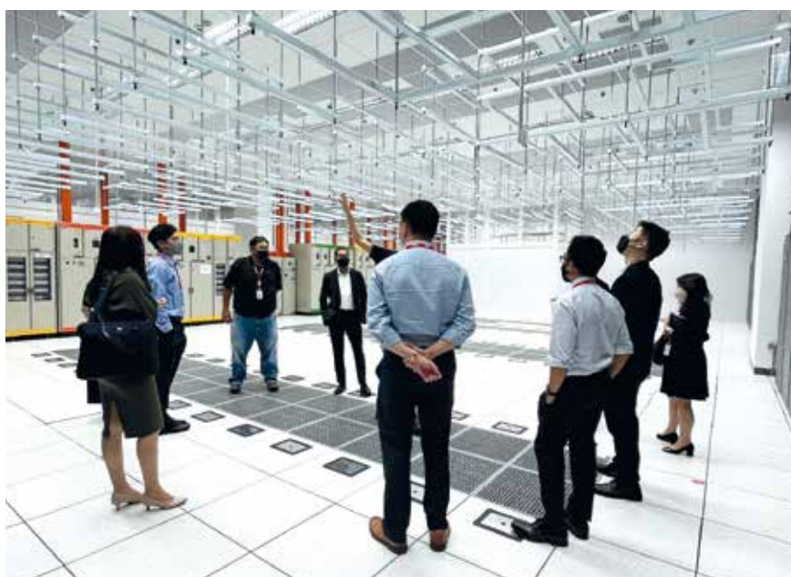
Investors at a data centre site visit.
