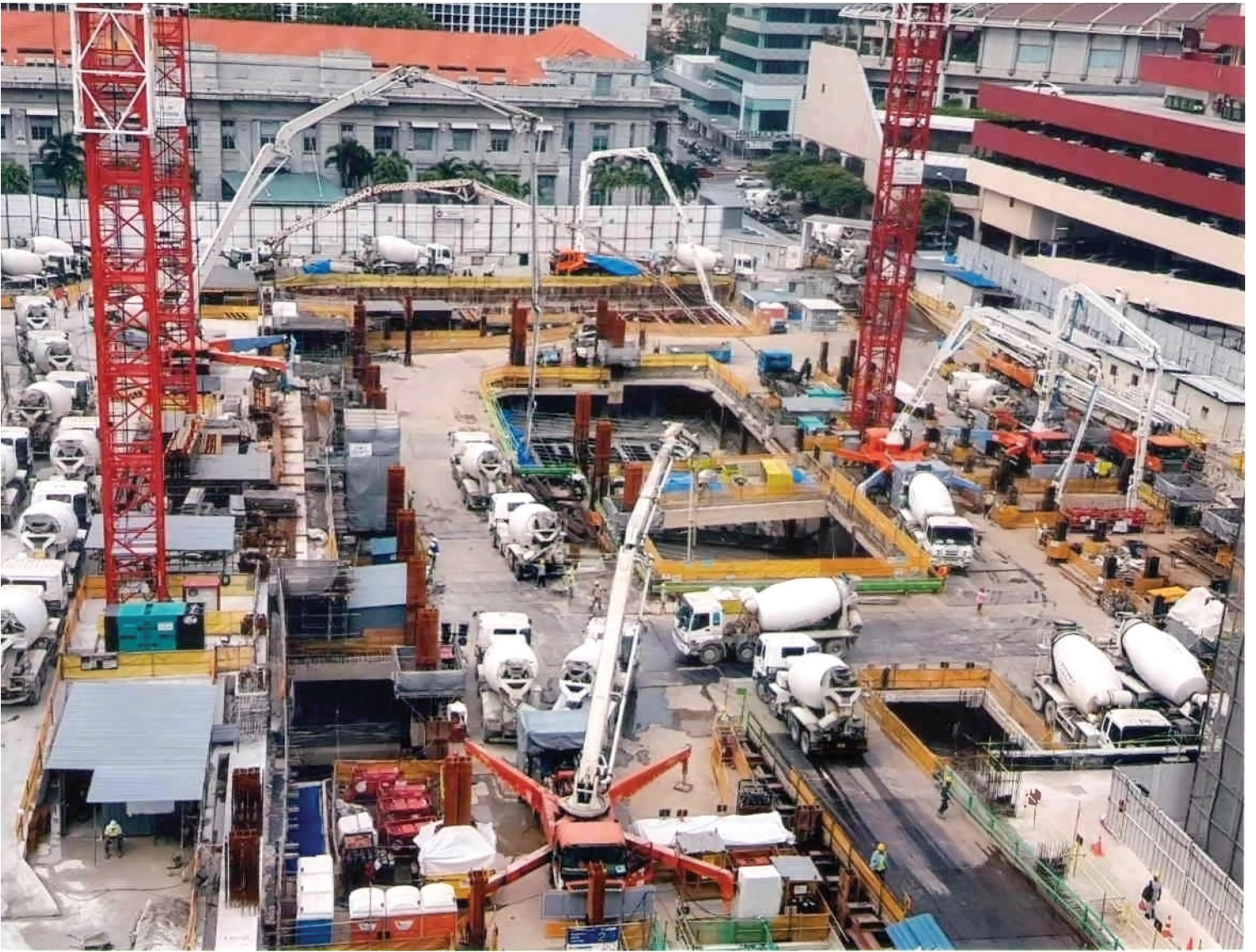
Concrete pumping equipment working on New State Courts Towers at Havelock Road
