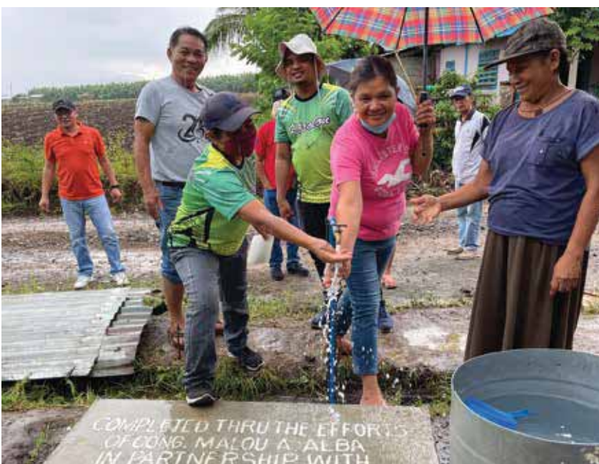
Water system installed in a community in Sumilao, Bukidnon
