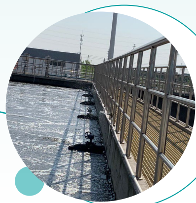
The biochemical pond spraying device at the sewage treatment plant
