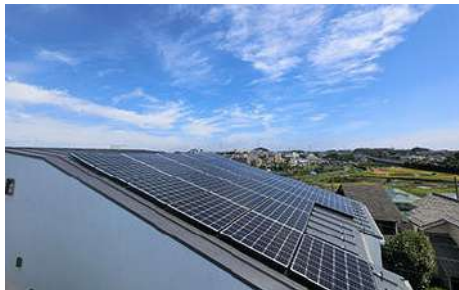
Solar power generation system
