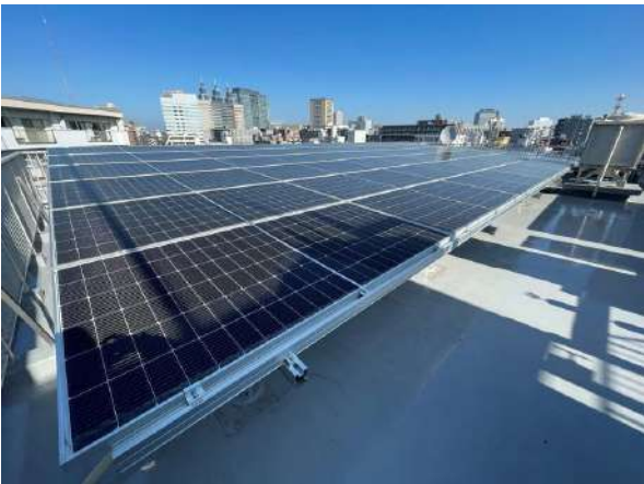
T's eco Kawasaki solar panels
