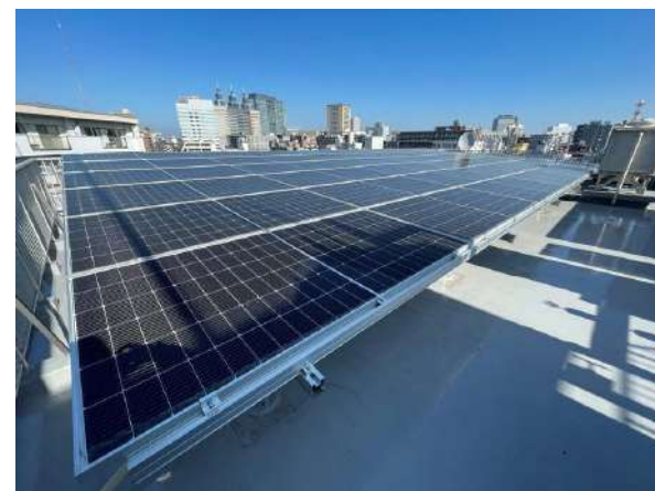
Solar panels installed on the rooftop
