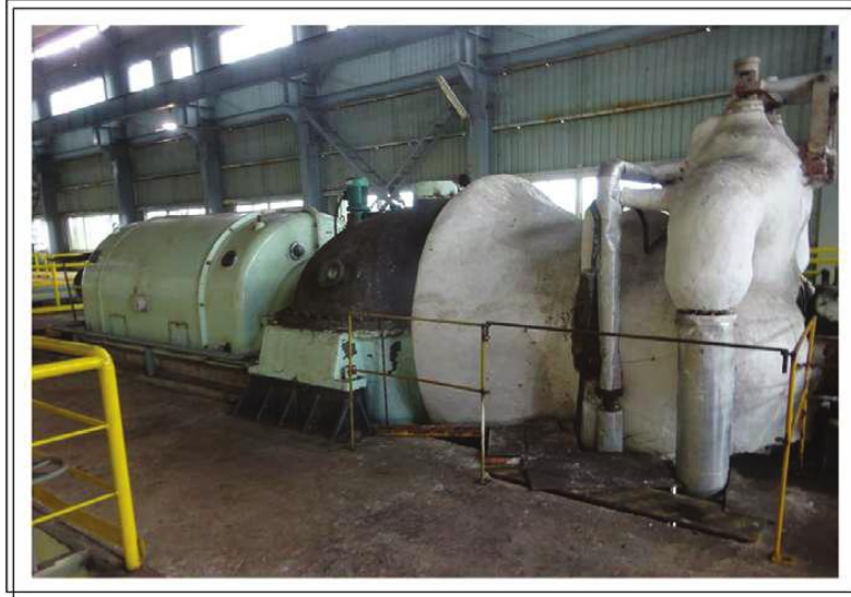
Engine Steam Turbine Generator 1 (2nd Floor)
