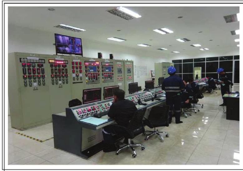
Room Control Panel
