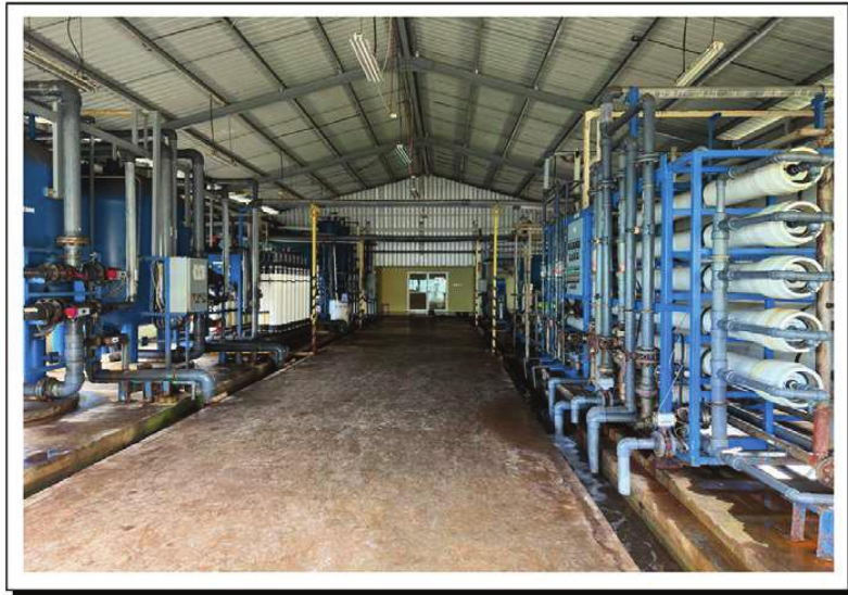
Laboratory and WTP : Inside View
