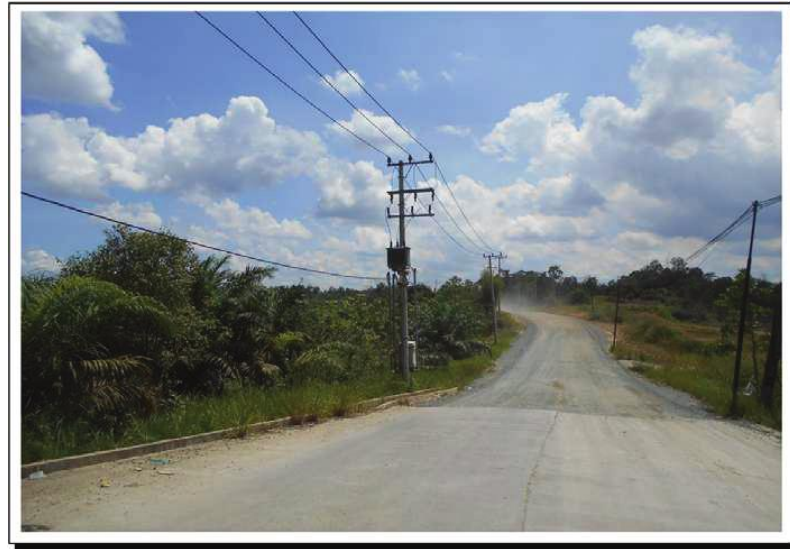
Distribusi Line 20 kV Concrete Poles & Transformers (From Substation to New Customer )
