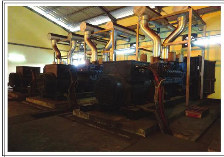
Diesel Power Plant
