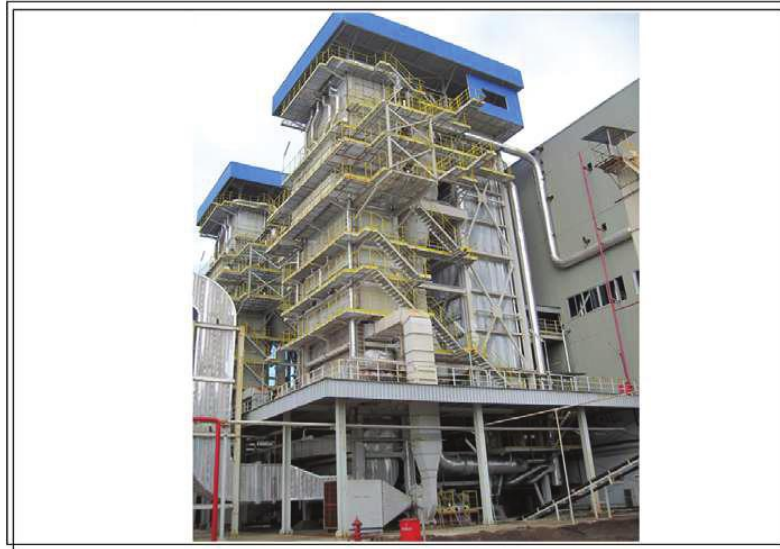
Circulating Fluidized Boiler 2
