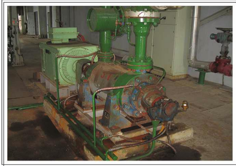
Boiler Feed Pump
