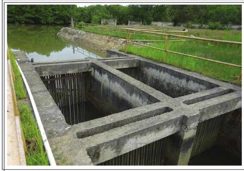
River Water Intake
