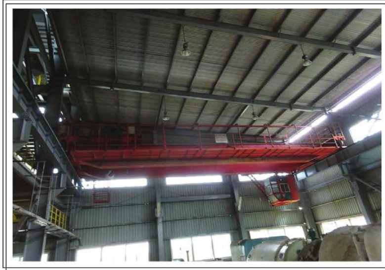
Over Head Traveling Crane
