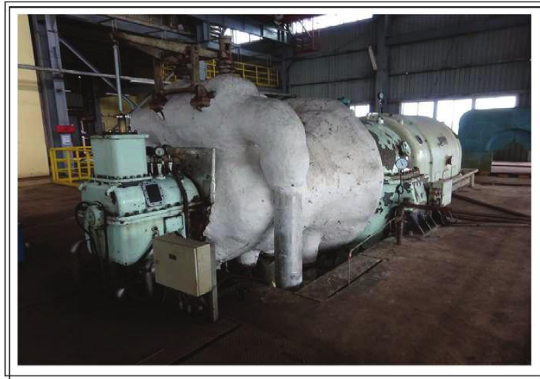
Engine Steam Turbine Generator 2 (2nd Floor)
