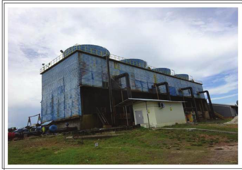
Cooling Tower System
