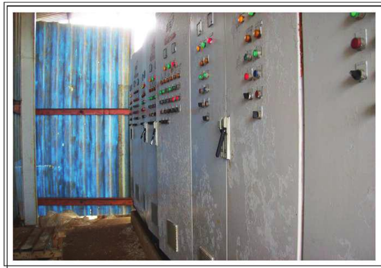
Cooling Tower PLC Panel
