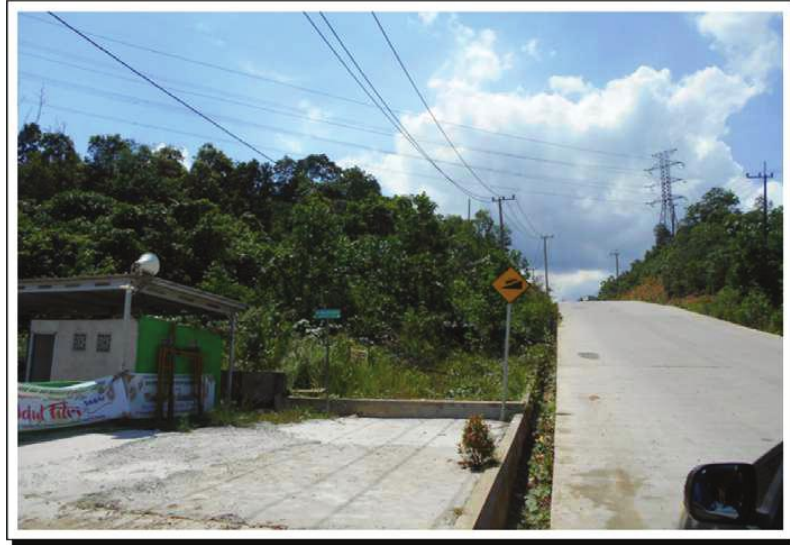
Distribusi Line 20 kV Concrete Pole (From Substation to new customer )
