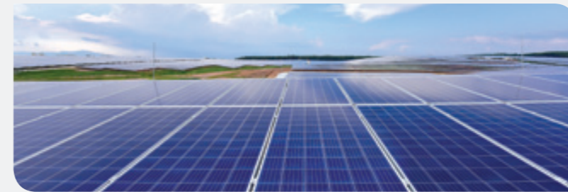
Solar Power Plant in Kuala Ketil, Malaysia.
