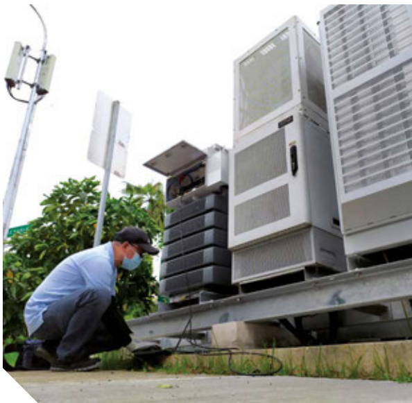
Engineer maintaining a mobile base station.
