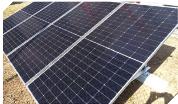
Photovoltaic panels producing electricity directly from sunlight to power our mobile base stations.
