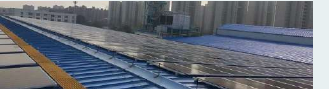
We adopt diverse technologies including rooftop solar panels to minimise our energy consumption across factories.
