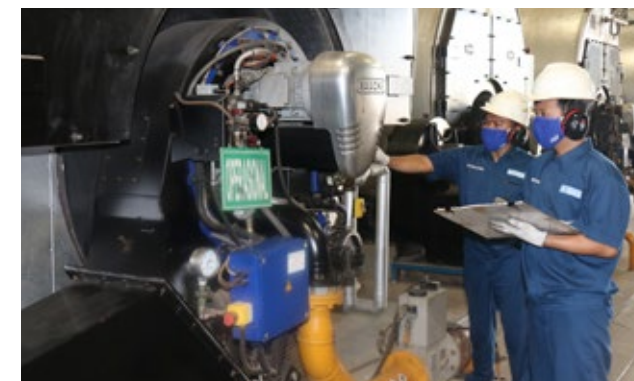
Energy consumption monitoring at the Priok Refinery, Jakarta.
