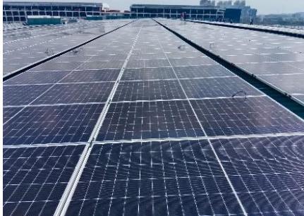
Solar PV system at 34 Penjuru Lane – operational since Feb 2024
