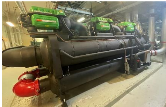
Upgraded air-conditioning chillers at 508 Chai Chee Lane – completed in Sept 2023
