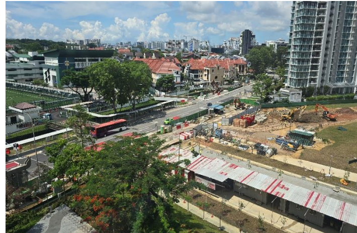
Aerial view of the ongoing infrastructure works, including road widening; photo taken in April 2024
