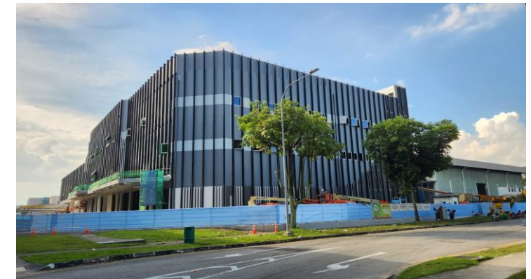
Sabana@1TA4 is targeted to obtain Temporary Occupation Permit around June 2024; Photo of Sabana@1TA4 taken in April 2024
