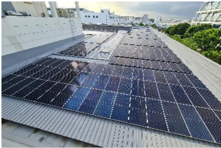
Solar PV system at 10 Changi South Street 2 – operational since Dec 2023
