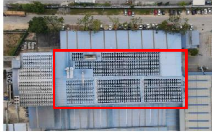
Lot 88, Rawang (1,636 kWp)
