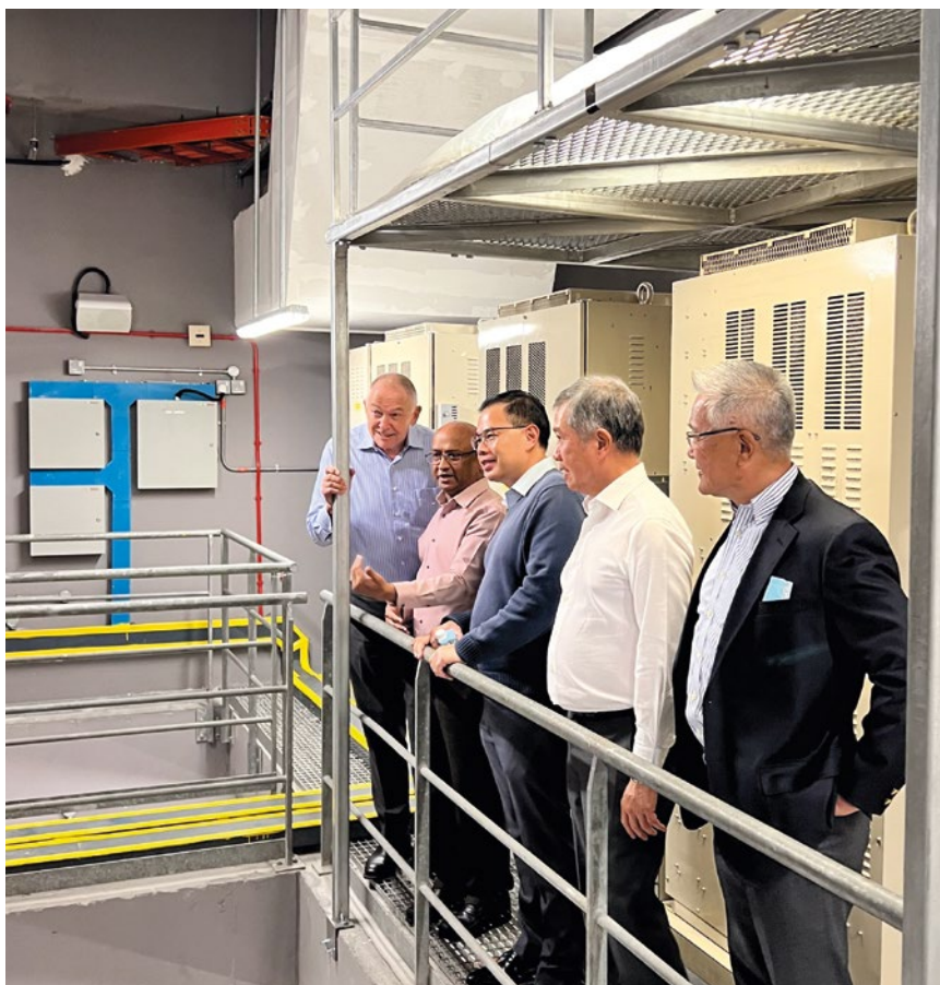
A safety walkabout was organised for the Independent Directors and management to inspect the safety features of Keppel REIT's properties in Singapore and observe how work was carried out on a day-to-day basis.
