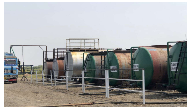
Jyoti I – Oil Storage
