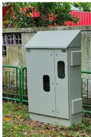
VOC Monitoring Unit
