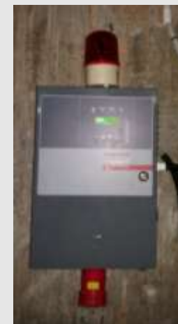
VSD for Condenser Water Pump
