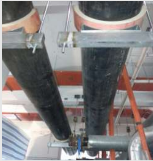
Chilled Water Pipe
