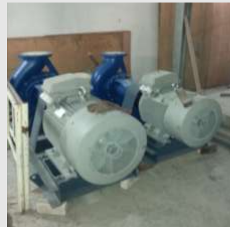
Chiller Water Pump and Condenser Water Pump
