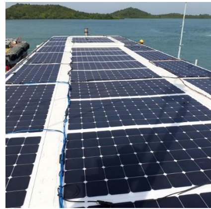
Close up of the solar panels installed
