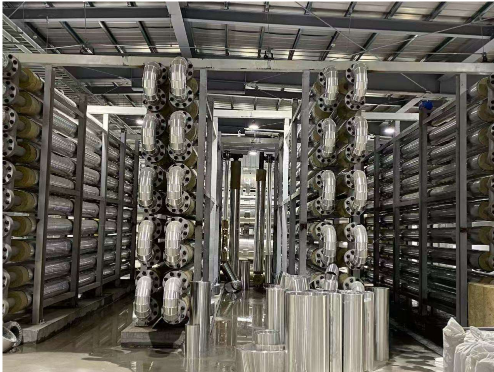
Sludge Treatment System Preheating Unit
