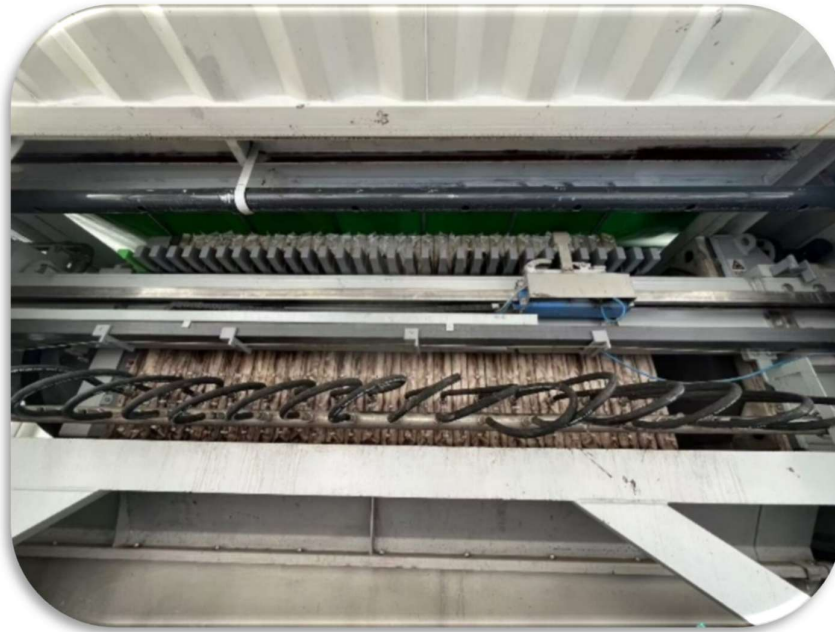
Sludge dewatering module, view from top
