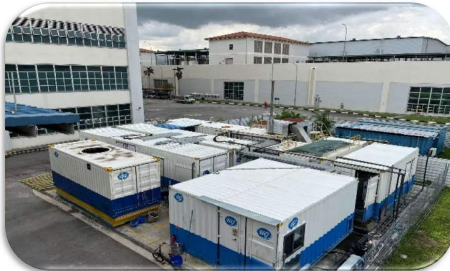
Sludge Treatment System housed in containerised modules at Changi Water Reclamation Plant
