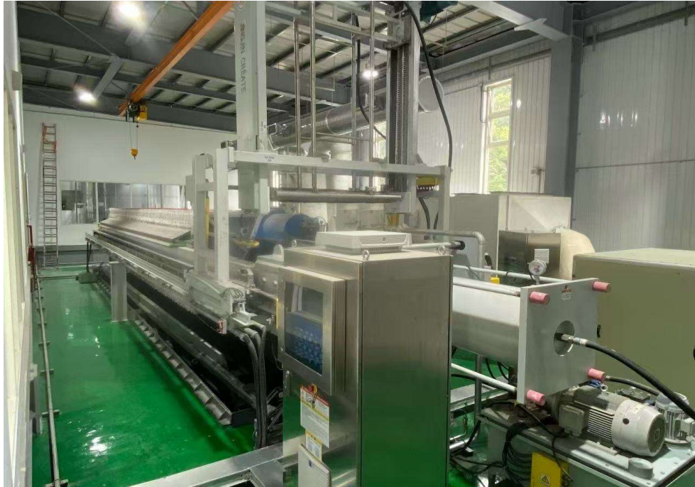
Sludge Treatment System Dewatering Unit
