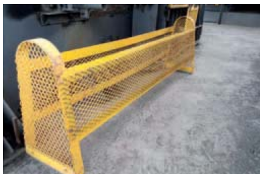
Mechanic guarding rectification
