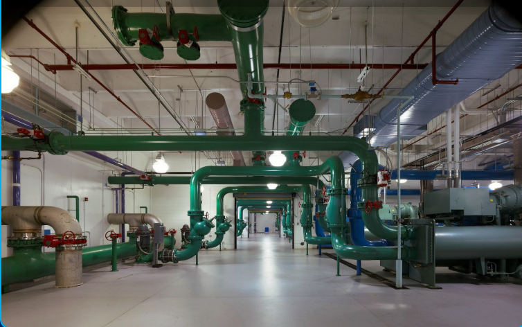
Dual Utility Water Feeds Enable AI Workloads
