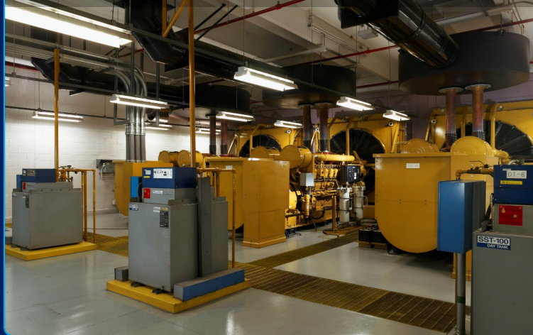
Prime-Rated Generators Support Resiliency
