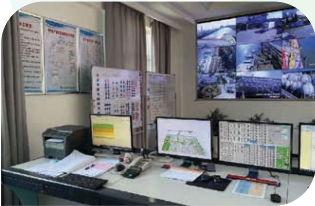
CENTRAL CONTROL ROOM
