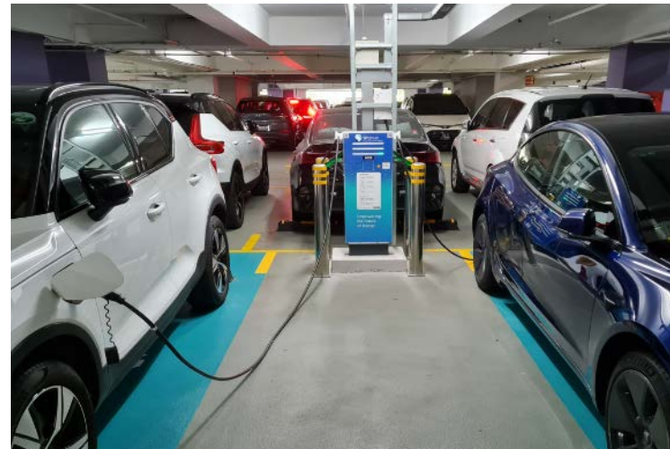
Electric vehicle charging points at United Square.
