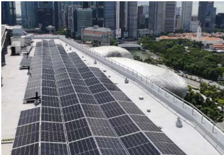
Solar panels were installed at the rooftop of PARKROYAL COLLECTION Marina Bay.
