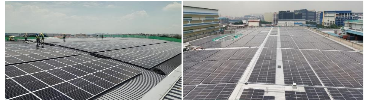
Solar panel installations at LogisTech and 40 Penjuru, Singapore
