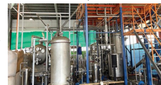
GEIH Processing facility
