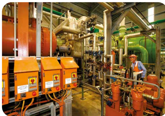
Cogeneration plant in Queensland, Australia.
