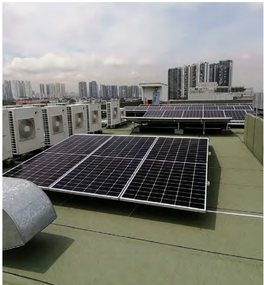
Figure 1: The Solar PV Systems at Mewah Headquarters, Singapore.
