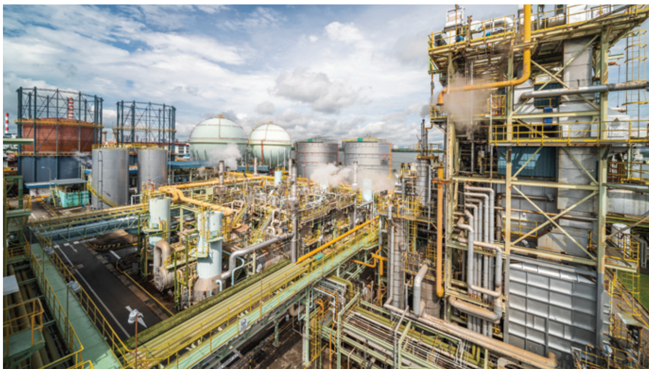
City Energy achieved 100% gas production availability at its Senoko Gasworks facility.
