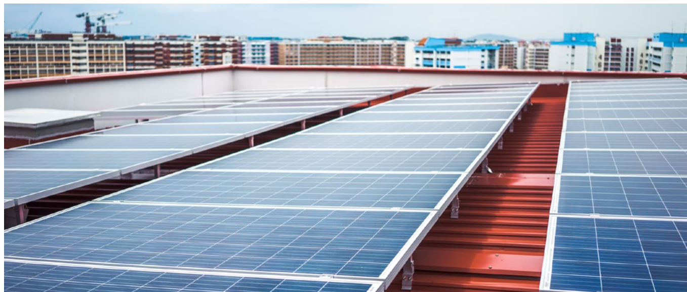
By 2020, more than 5,500 HDB blocks would be installed with solar photovoltaic panels
