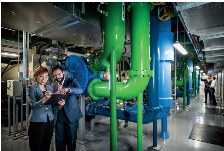
Keppel's integrated ecosystem for digital infrastructure combines fund management and investment expertise with deep operational capabilities. (In picture: A data centre cooling system at the Keppel Data Centre Campus.)
