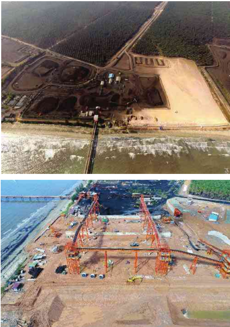
Figure 9:5 Coal Loading Facilities at Port
