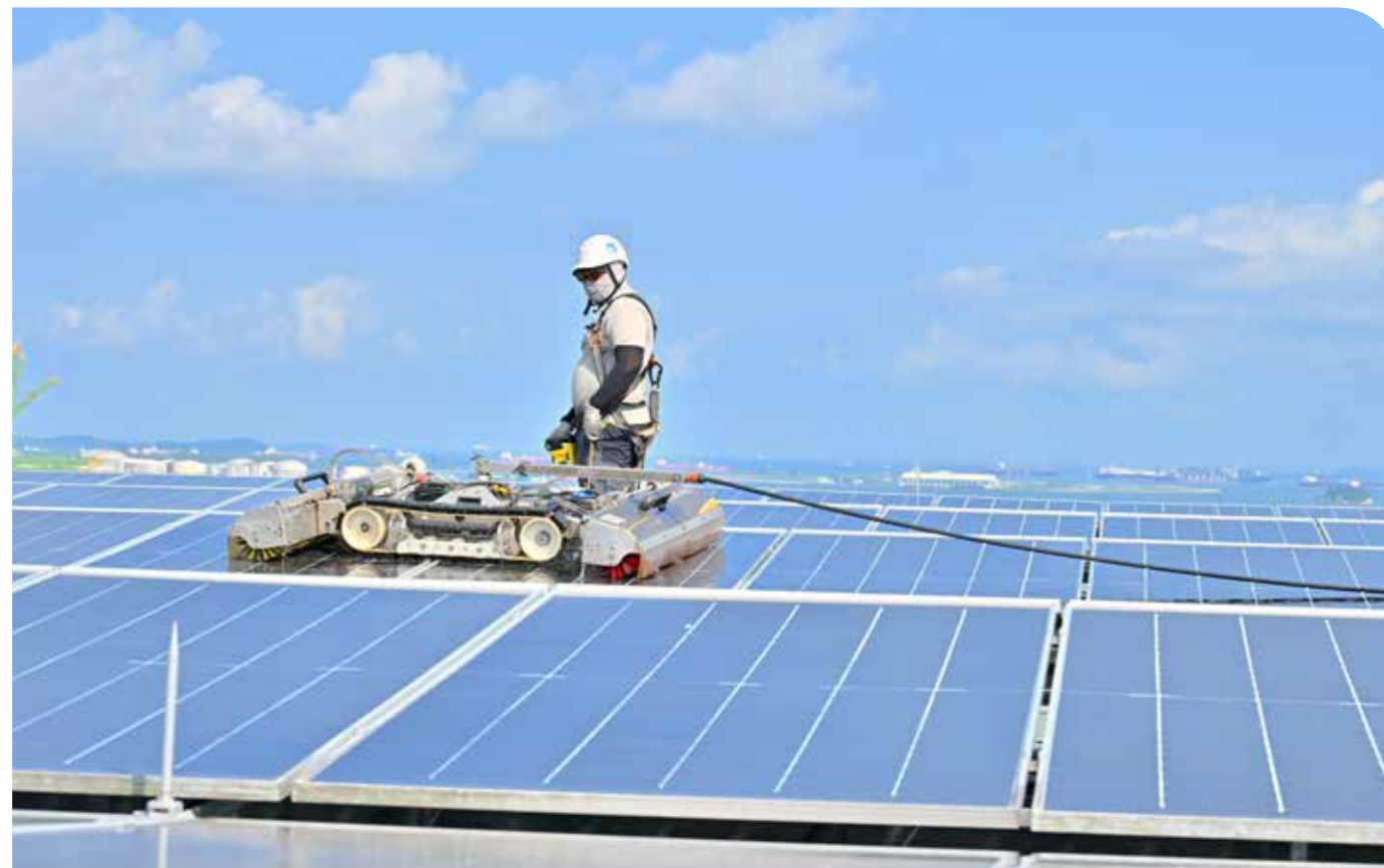
Solar panels at MBC undergoing routine cleaning and maintenance.
